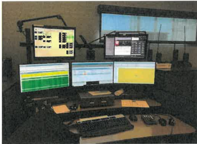
Figure 3: CONFIRE ECC Console Arrangement
