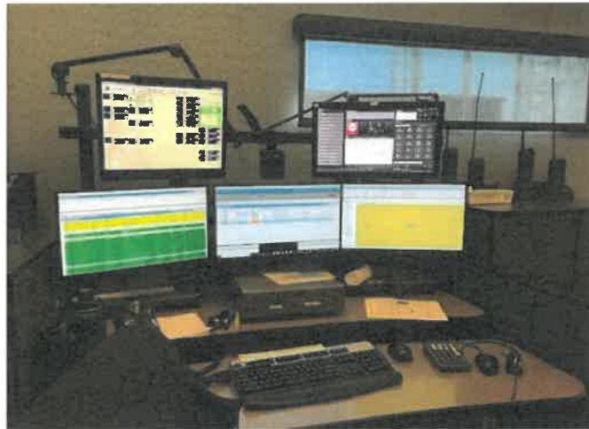
Figure 3: CONFIRE ECC Console Arrangement
